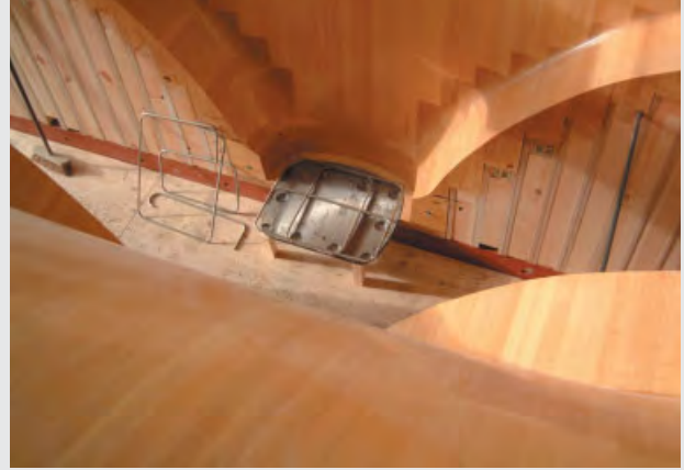
The 'foot' of the Ballingdon Bridge pier mould split at Buchan's works in Lancashire, ready for installation of the reinforcement.
