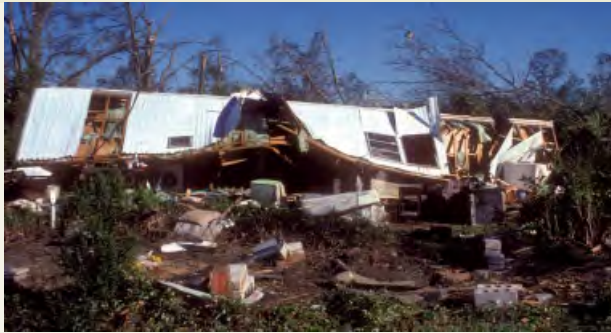
A mobile home following the attentions of a tornado in Alabama, us. The loss of life and property from the use of unsuitable and unsustainable timber structures is endemic. The economic calculations involved in making houses in the cheapest and fastest manner, using the minimum of labour and materials, are formidable. It is difficult to redirect this economic leviathan towards another way to produce human habitation.
