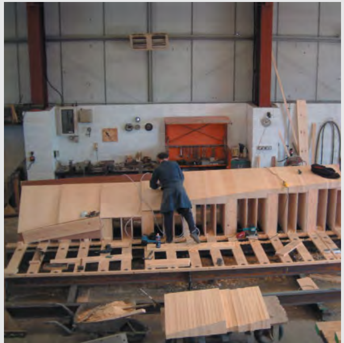
One of the precast-concrete models of Ballingdon Bridge under construction at Buchan's works in the West Midlands.
