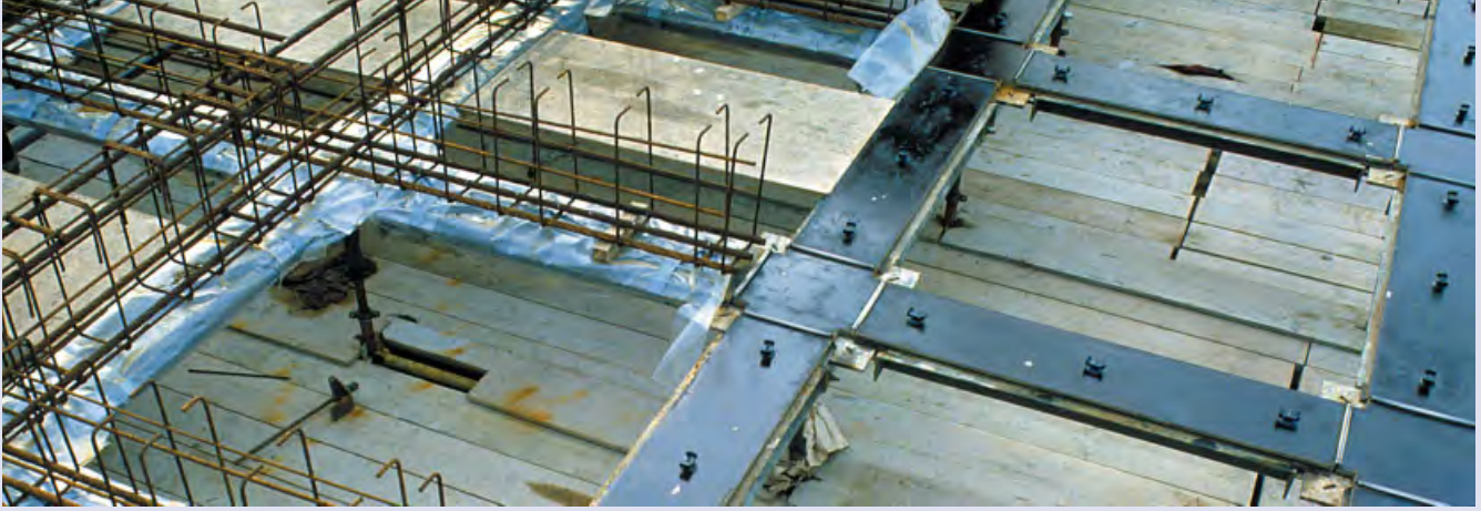
A section of assembled soffit forms showing the reinforcement support cradles for the Lloyd's floors. The raised strips at the intersections are the steel channels which contain the gaskets for the node/beam joints.
