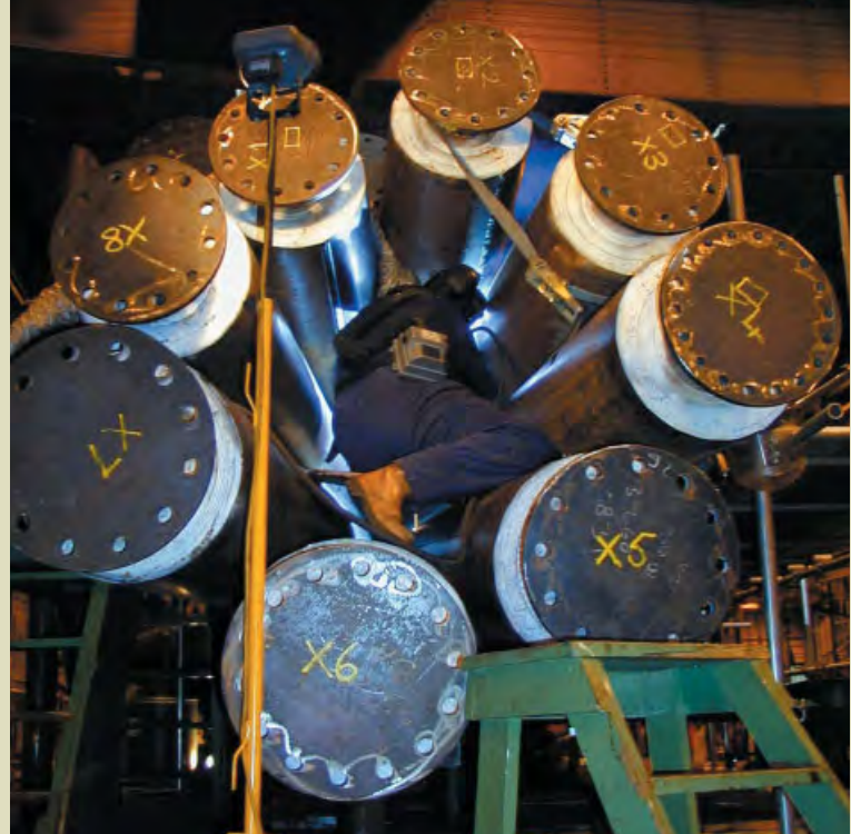
Figure 6: Specialists. Some of the welds required left-handed welders using modified welding equipment, simply to get at the more 'embedded' welds.
