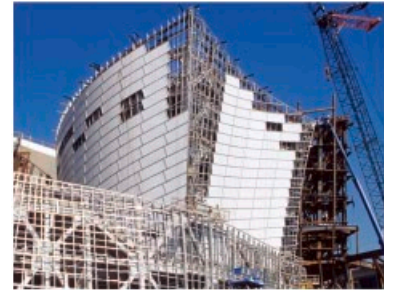
Figure 2. Gehry Partners, Walt Disney Concert Hall, Los Angeles, 2002 The enclosure detailing connects features from two distinct mappings between 2-D and 3-D space: the ruling lines of the global developable surface, and a patterning of lines in the unfolded surface space, injected back into 3-D space as geodesic curves.
